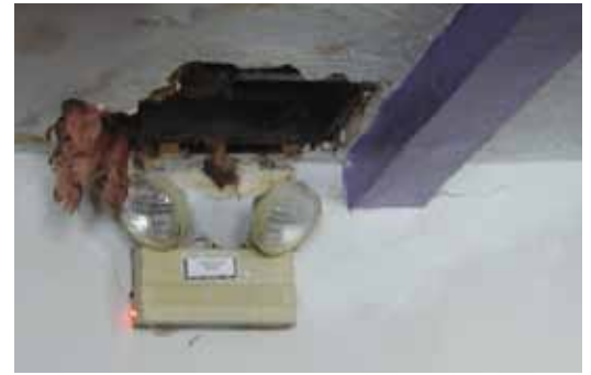
Hole in classroom ceiling
