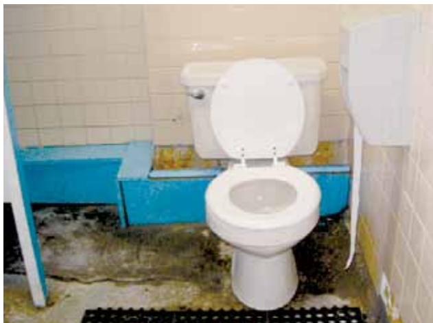
Rough concrete floor and leaky toilet
